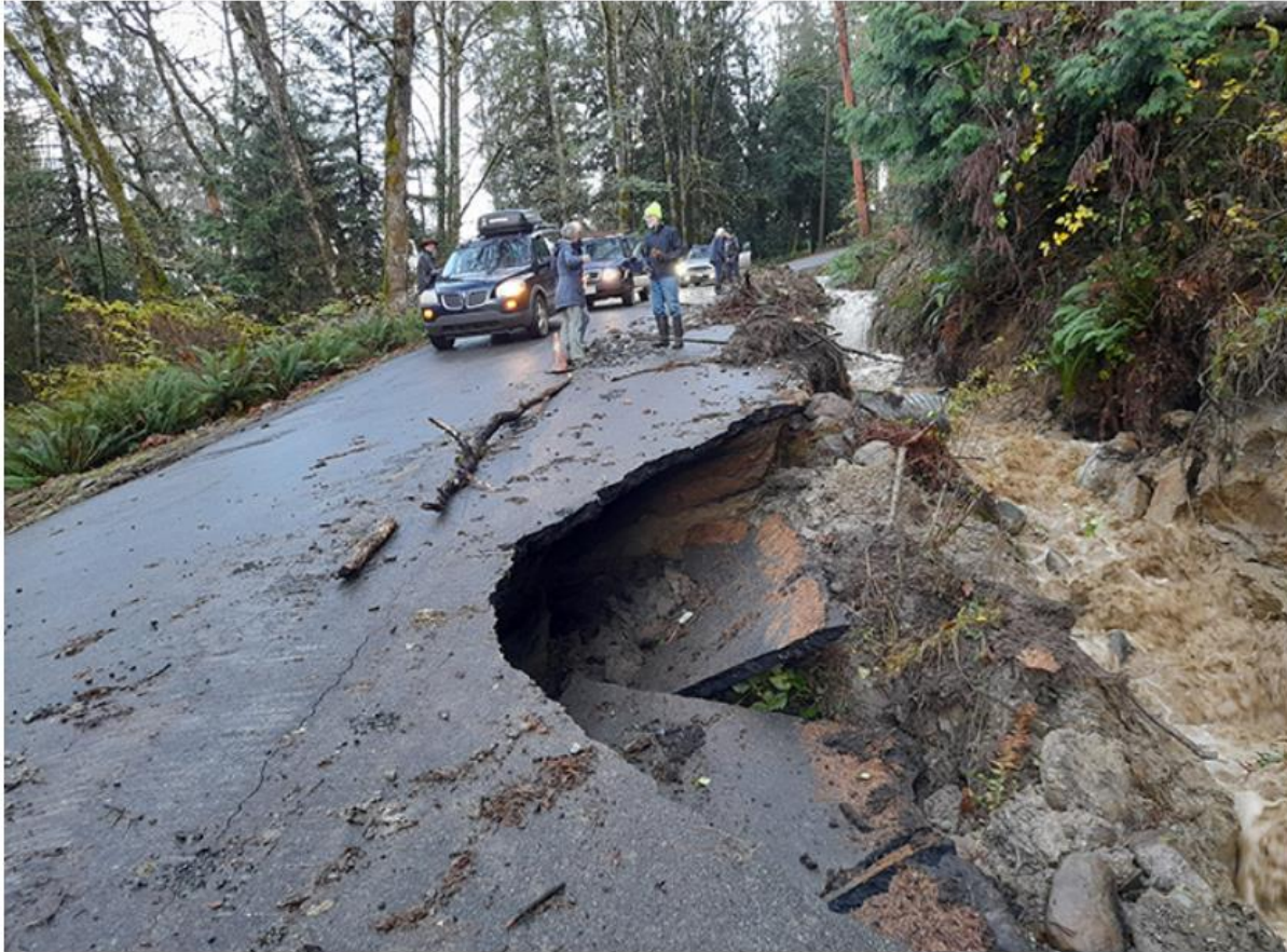
Damage in the form of a washout and erosion caused by heavy rains at the junction of Roland Road and Isabella Point Road at 3 p.m. on Nov. 15.
