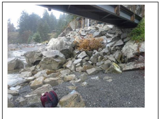
Shoreline sediment processes interrupted by riprap/boulders Photo: RC de Graaf
