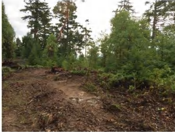
Photo 2: Area disturbed as part of construction of the new development. Once the new development is complete, this area should be replanted with any of the native groundcover plants listed in this report, or with grass seed to re-stabilize the soils and prevent invasive species such as Scotch broom and Himalayan blackberry from populating the site. Grass will help to stabilize the soils on the surface, however its relatively shallow roots will not provide as much stability and complexity as small shrubs and native groundcover plants.
