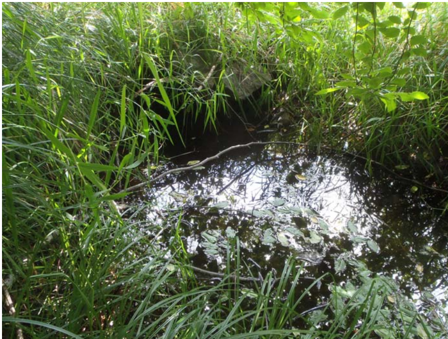
Photo 2. Water upstream of the culvert. Note deteriorated condition of the culvert.
