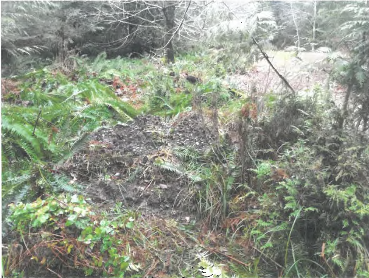
Photo 9: Soils removed from Valens' Brook during initial installation of two 0.45 m culverts that have been sidecast onto riparian vegetation. These materials should be removed and replaced into the streambed to fill the channel and pool created by the newly installed culverts (Photo 2) and/or spread thinly into surrounding riparian vegetation so as not to suffocate existing plants. The area underneath the soil pile should be replanted as needed.
