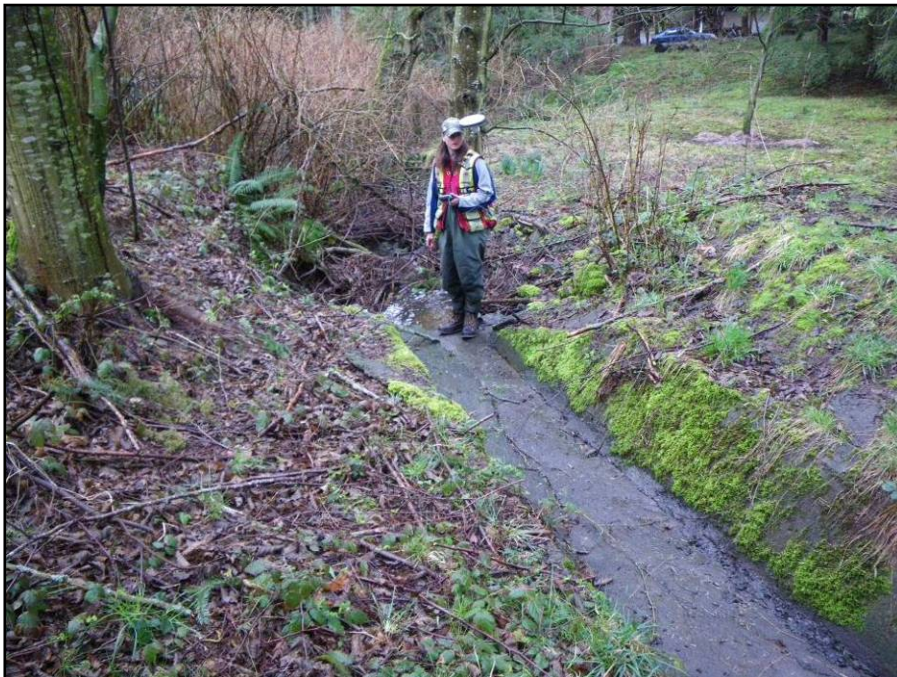
Looking down the concrete pond overflow. During the assessment, water was flowing underneath the flume.
