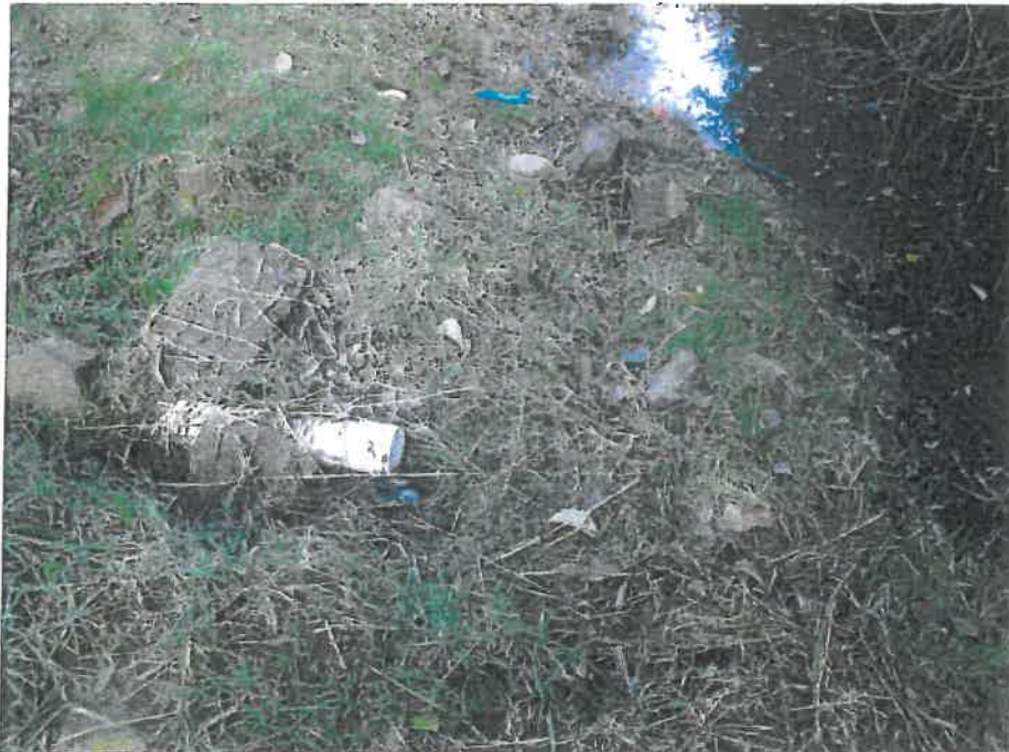
Outlet of perforated pipe connected to perimeter drains around the residence.
