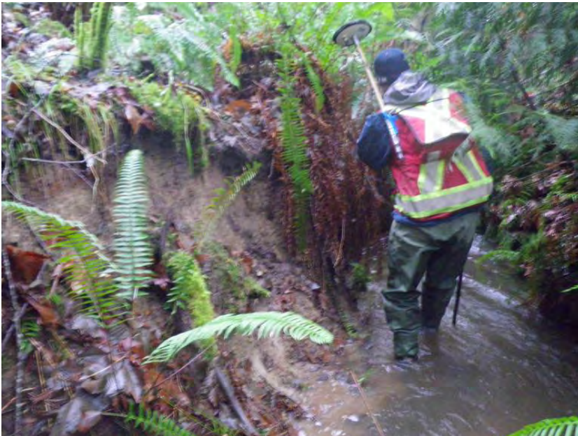
Typical over-steepened banks associated with historical channel straightening on Castell Brook.
