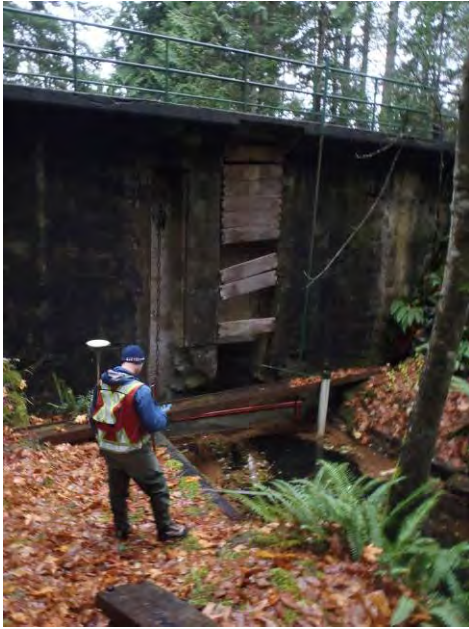
Looking at the upstream side of the dam and weir structure which backs up water on Hoggan Creek for hydro-electric power generation.
