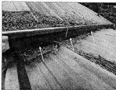
Previous Repair Noted
