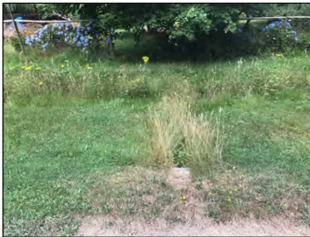
Photo 3. A 30cm diameter crossing Wildwood Crescent feeds the watercourse fronting the subject parcel from the roadside ditch on the east side of the road.
