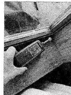
Moisture Noted At Window
