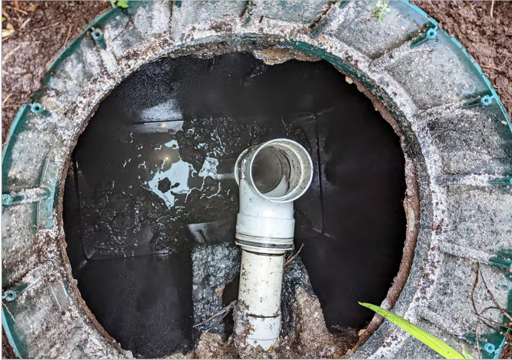
Picture 4: Outlet baffle (no filter installed)
