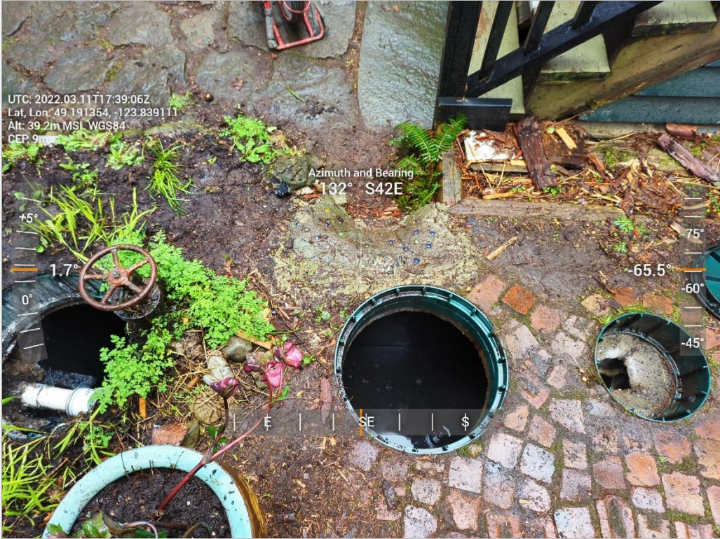
Picture 2: GPS location of septic tank (shows 3 access openings)
