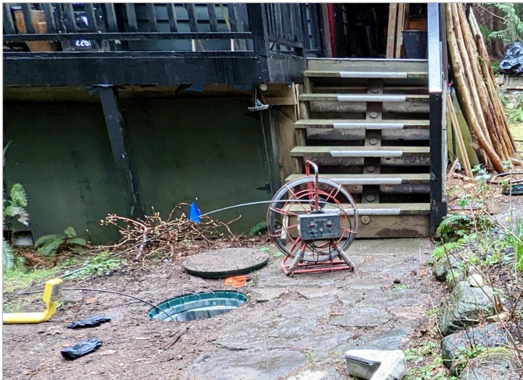
Picture 5: Location of distribution box (d-box)
