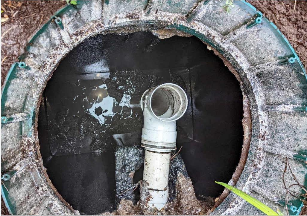
Picture 4: Outlet baffle (no filter installed)
