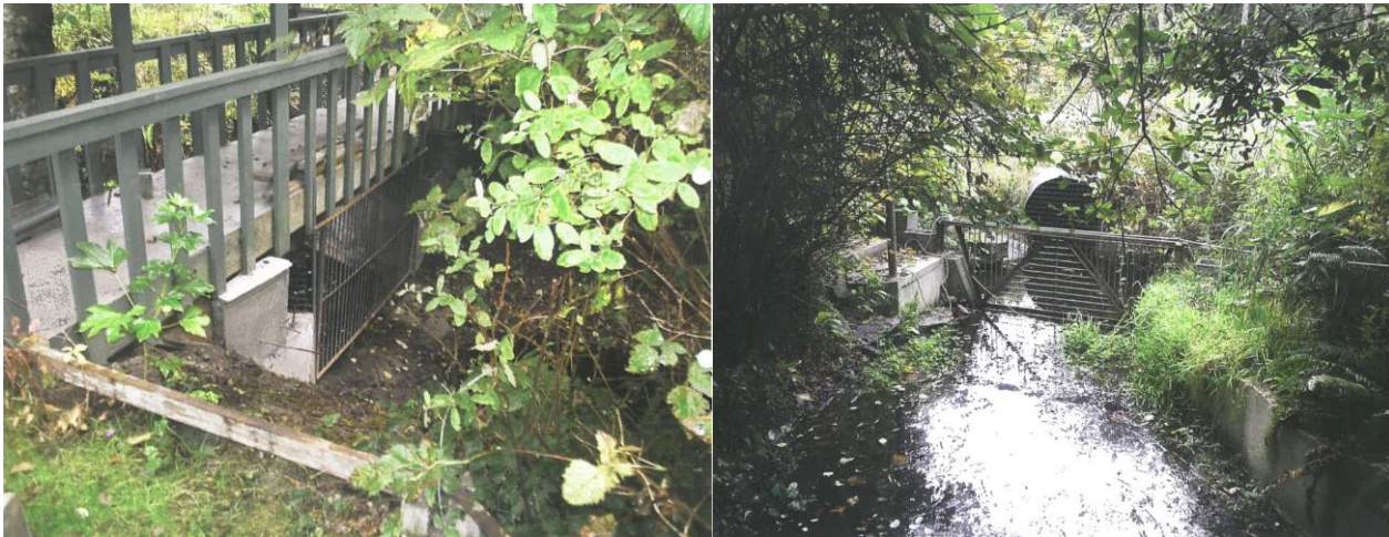
Bylaw enforcement staff initial site investigation photos taken in 2010, showing concrete bridge abutments, metal grates (since removed), and concrete channel hardening.
