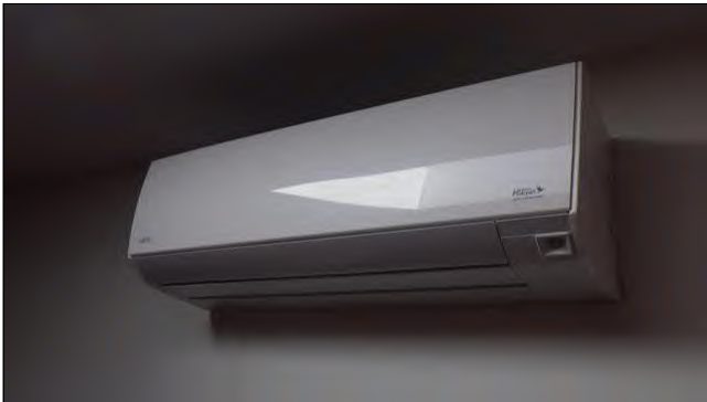
11.2 INDOOR BLOWER / FAN (Picture 3)
