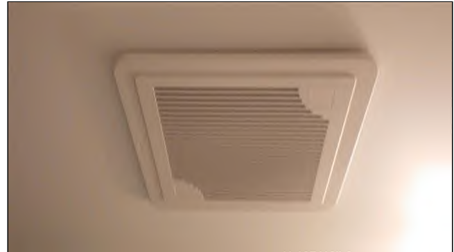
5.7.B VENTILATION (Picture 1)
