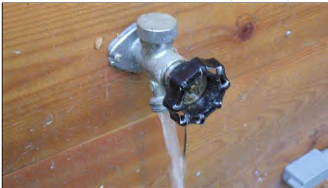
12.4 EXTERIOR FAUCET(S) (Picture 2)
