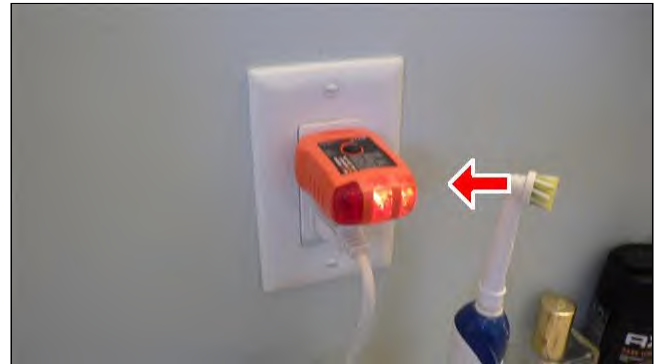
5.8.A ELECTRIC / GFCI (Picture 1)
