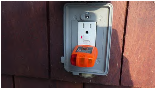
2.6 ELECTRIC / GFCI (Picture 1)
