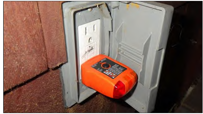
2.6 ELECTRIC / GFCI (Picture 2)
