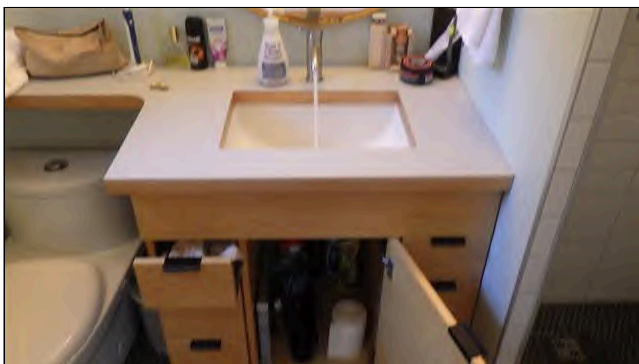
5.0.A SINK(S) (Picture 1)
