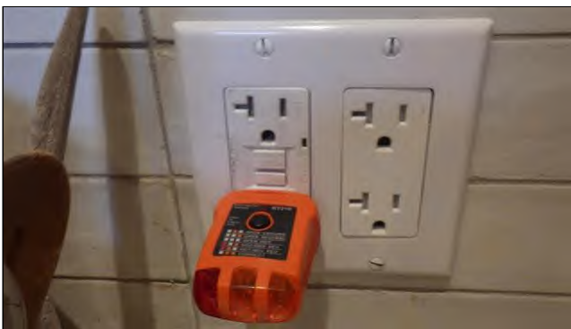
6.9 ELECTRIC / GFCI (Picture 1)
