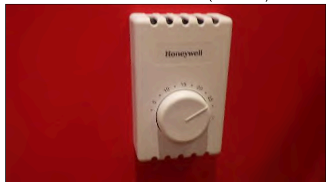
10.1 HEATING UNIT #2 (Picture 4)
