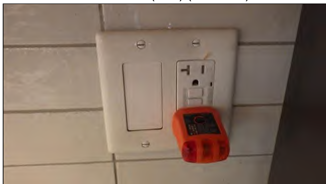
6.9 ELECTRIC / GFCI (Picture 2)
