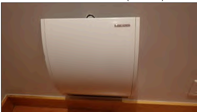
10.1 HEATING UNIT #2 (Picture 3)
