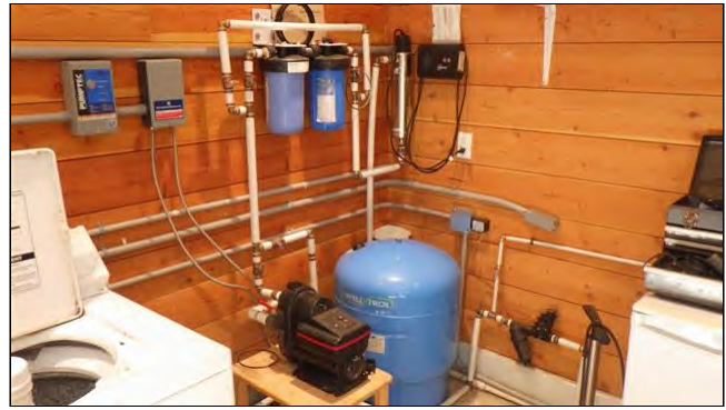
12.0 WATER PIPING (Picture 4)
