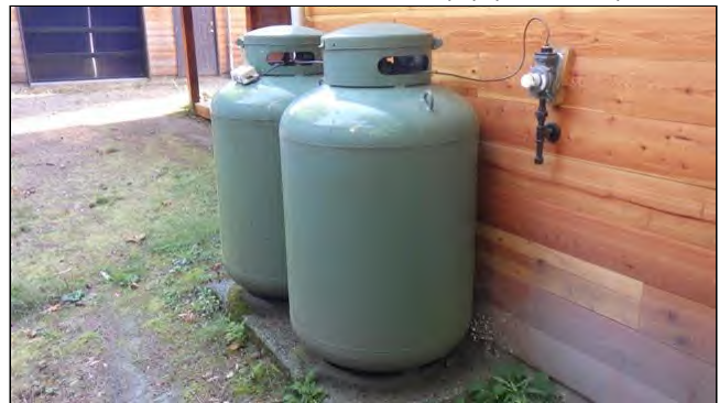
12.5 GAS PIPING (Picture 1)
