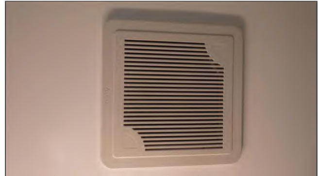
5.7.A VENTILATION (Picture 1)
