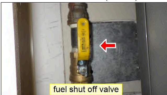
13.2 GAS / FUEL LINES AT UNIT (Picture 1)
