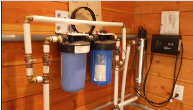
12.0 WATER PIPING (Picture 5)
