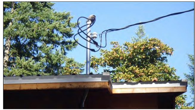
9.0 SERVICE / ENTRANCE LINE (Picture 2)
