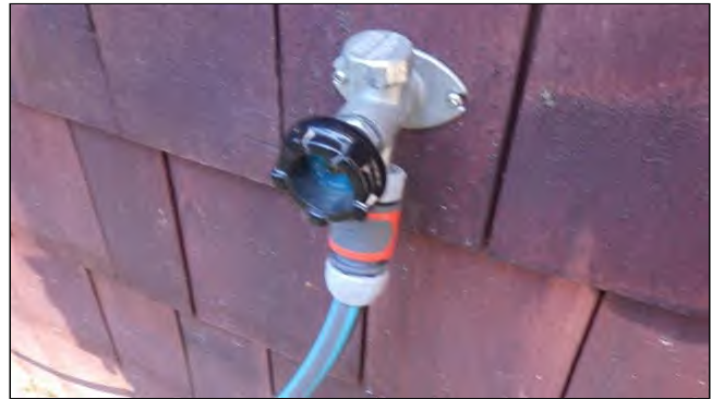
12.4 EXTERIOR FAUCET(S) (Picture 1)
