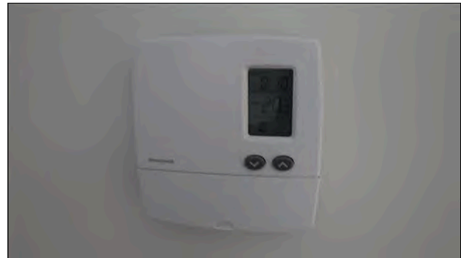
10.1 HEATING UNIT #2 (Picture 2)
