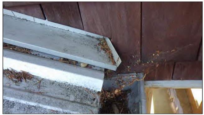
1.6 EXPOSED FLASHING (Picture 2)
