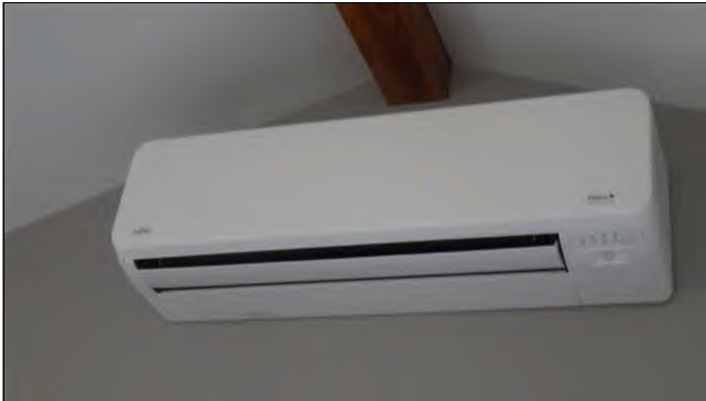
11.2 INDOOR BLOWER / FAN (Picture 1)
