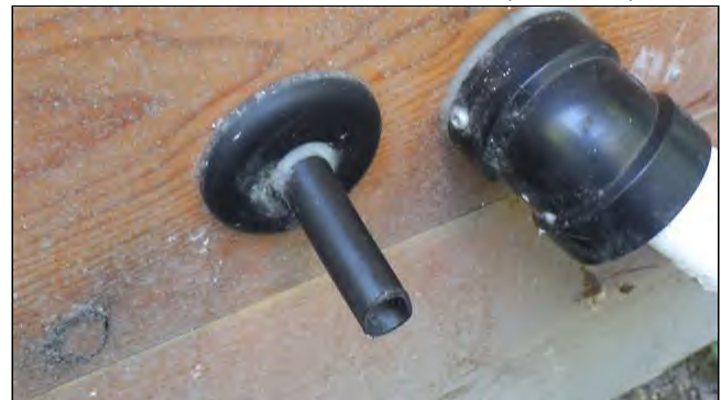
11.3 CONDENSATE PROVISIONS (Picture 2)
