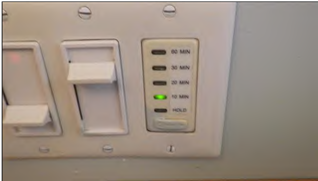
5.7.A VENTILATION (Picture 2)
