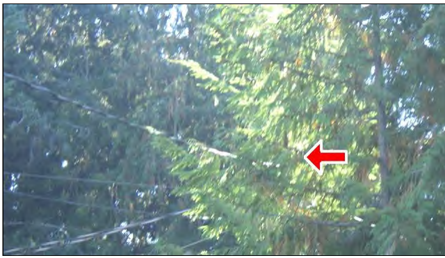
9.0 SERVICE / ENTRANCE LINE (Picture 1)
