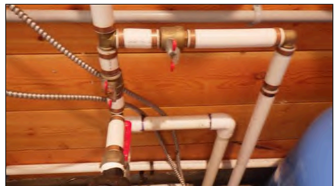
12.0 WATER PIPING (Picture 2)
