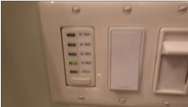
5.7.B VENTILATION (Picture 2)
