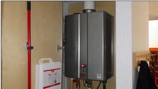
13.0 WATER HEATER (Picture 1)
