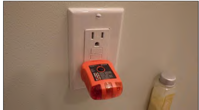
5.8.B ELECTRIC / GFCI (Picture 1)
