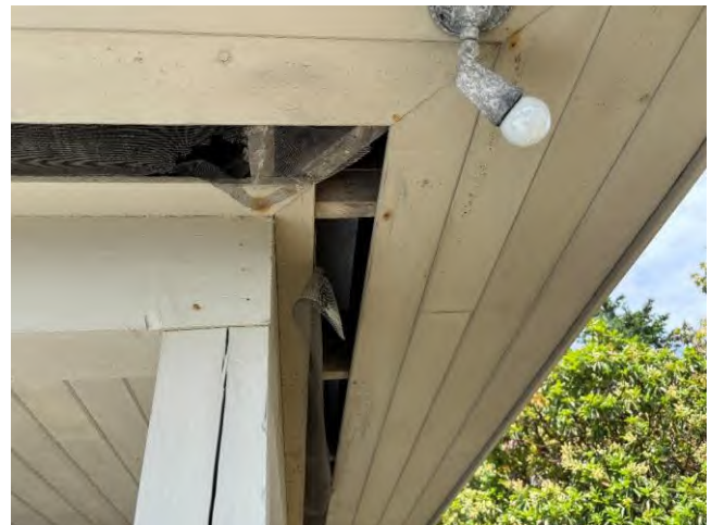
Photo 12: View of missing exclusion mesh under the eaves and potential access location for small wildlife (May 27, 2025).
