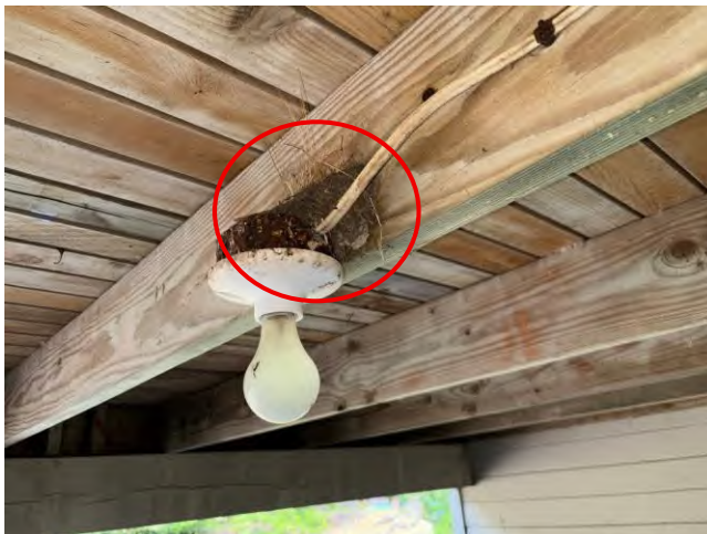
Photo 11: View of unoccupied barn swallow nest (red circle) on light fixture in the carport area (May 27, 2025).
