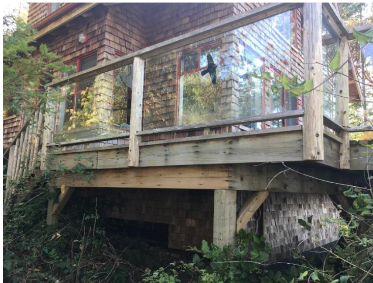
PHOTO 1. SIDE VIEW OF DECK AND HOUSE AT LOCATION OF SETBACK ENCROACHMENT
