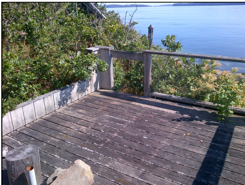
Picture 1 – Deck surface with tree growing through
