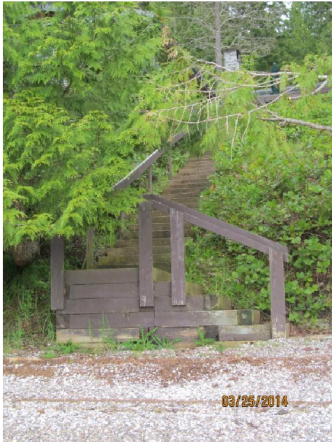
Picture 1: Non-compliant stairway to the beach
