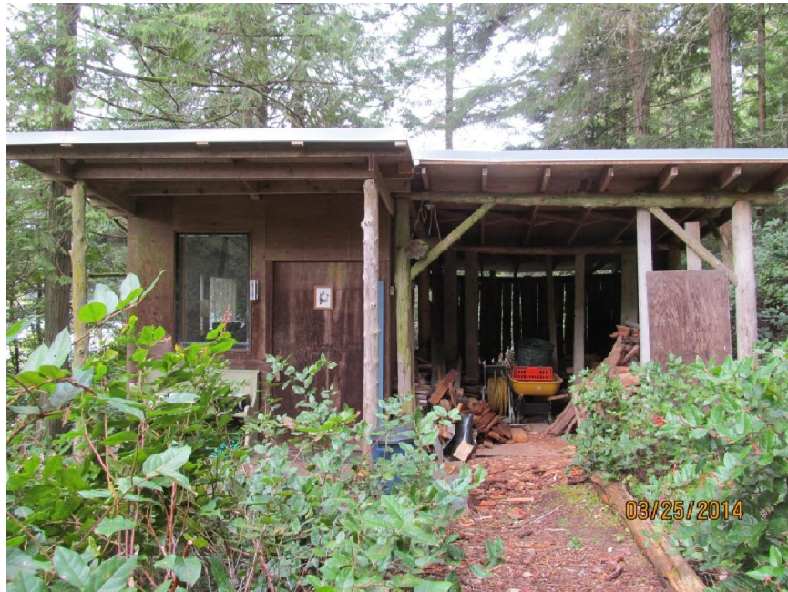
Picture 3: Non-compliant shed (north side of lot)
