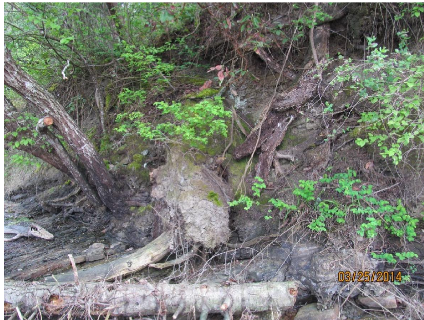
Picture 4: Shoreline erosion
