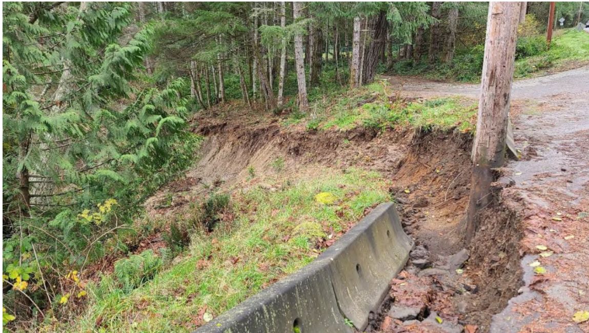
Photo 15: Shows the landslide and some of the damage to Sturdies Bay Road.
