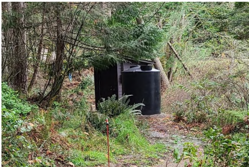
Photo 14: Shows the pumphouse and water tank.
