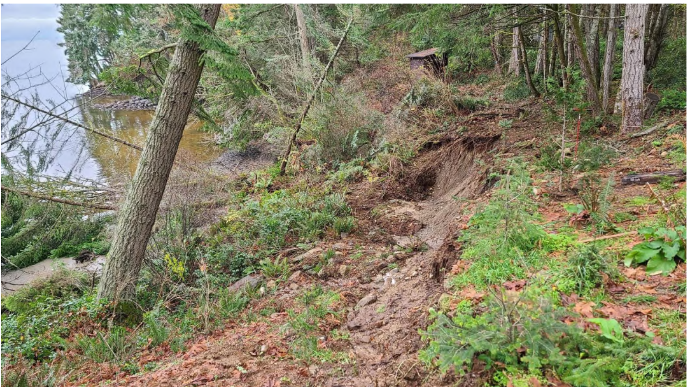
Photo 7: Shows the landslide down into Murcheson Cove and state of vegetation. Also illustrates the 'face' of exposed soil along with the intact utility trench (under the red soil probe on right of photo).
