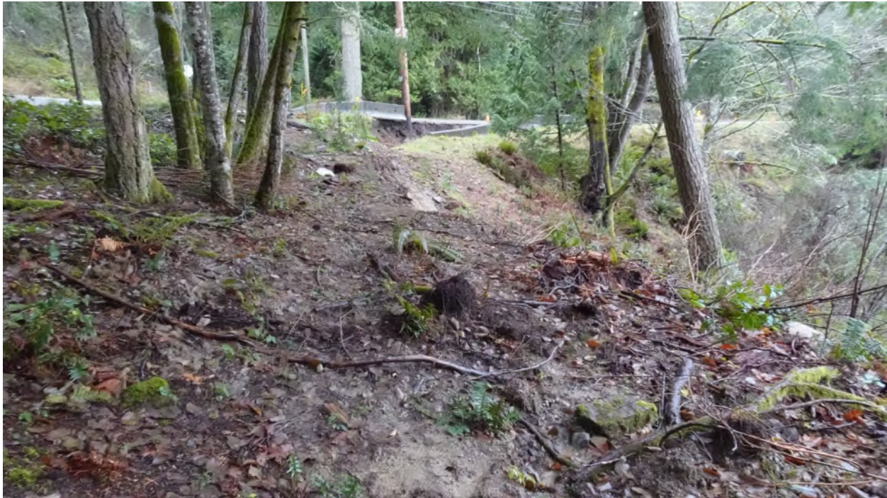
Photo 2 – View from the pump house towards Sturdies Bay Road. The trench for the water line and power line was adjacent to the trees on the left. Note new vegetation that has been placed near Sturdies Bay Road. Vegetation debris lays across the trench location.
