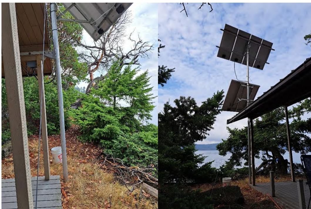
LEFT: LOOKING SOUTHEAST (DECK, SOLAR PANEL) RIGHT: LOOKING SOUTHWEST (DECK, SOLAR PANEL)
