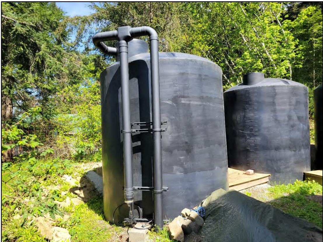
WATER TANKS, LOOKING NORTH
