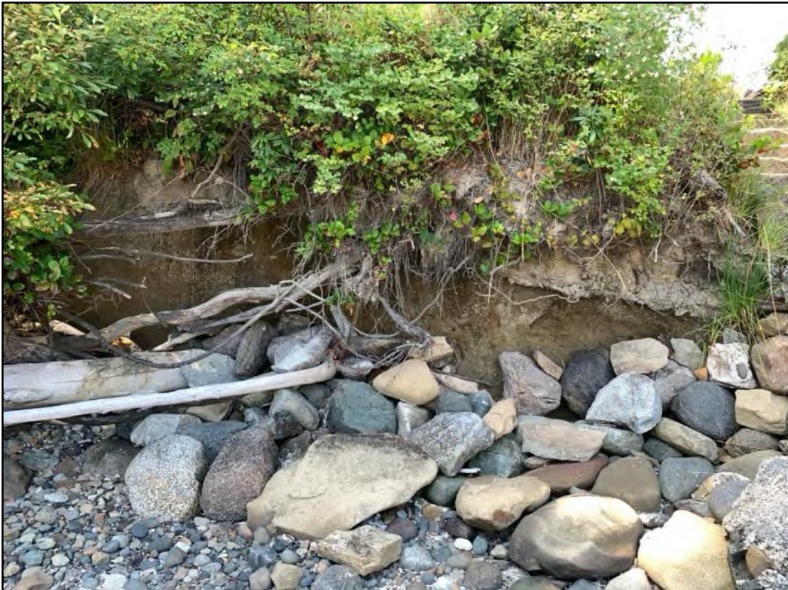
SHORELINE EROSION, LOOKING WEST
