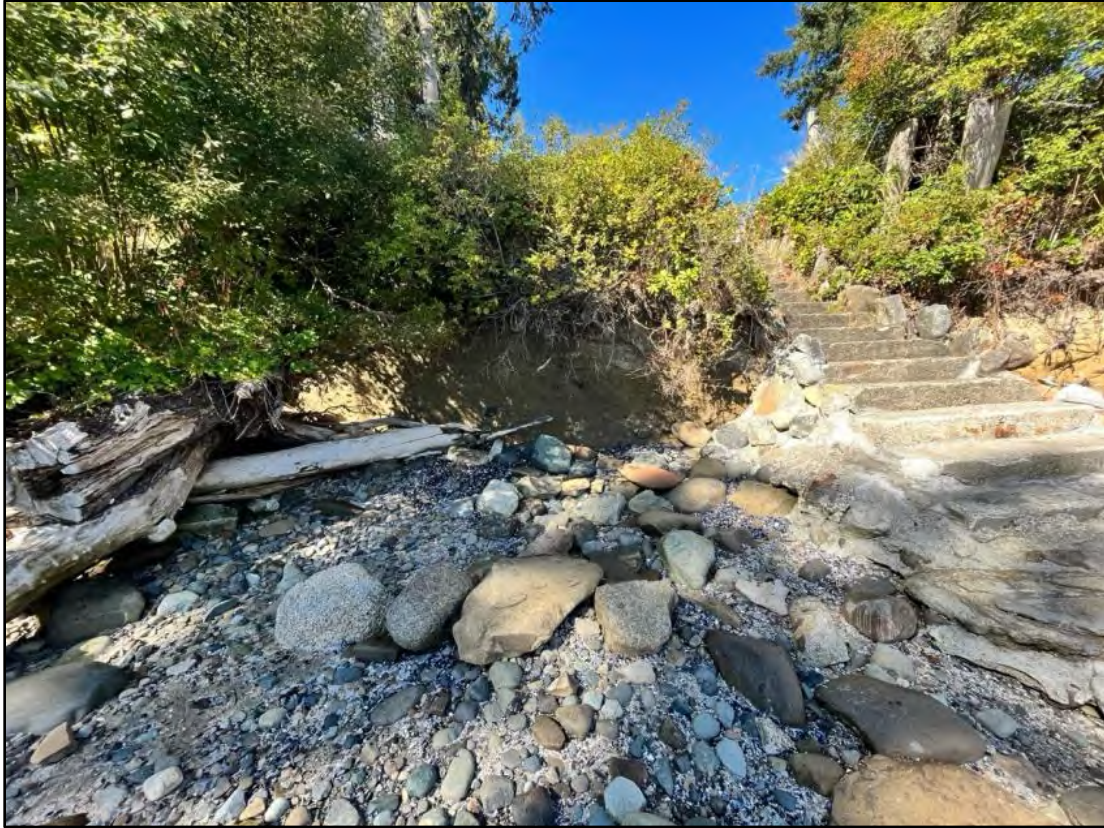
EXISTING STAIRS AND BANK EROSION, LOOKING WEST
