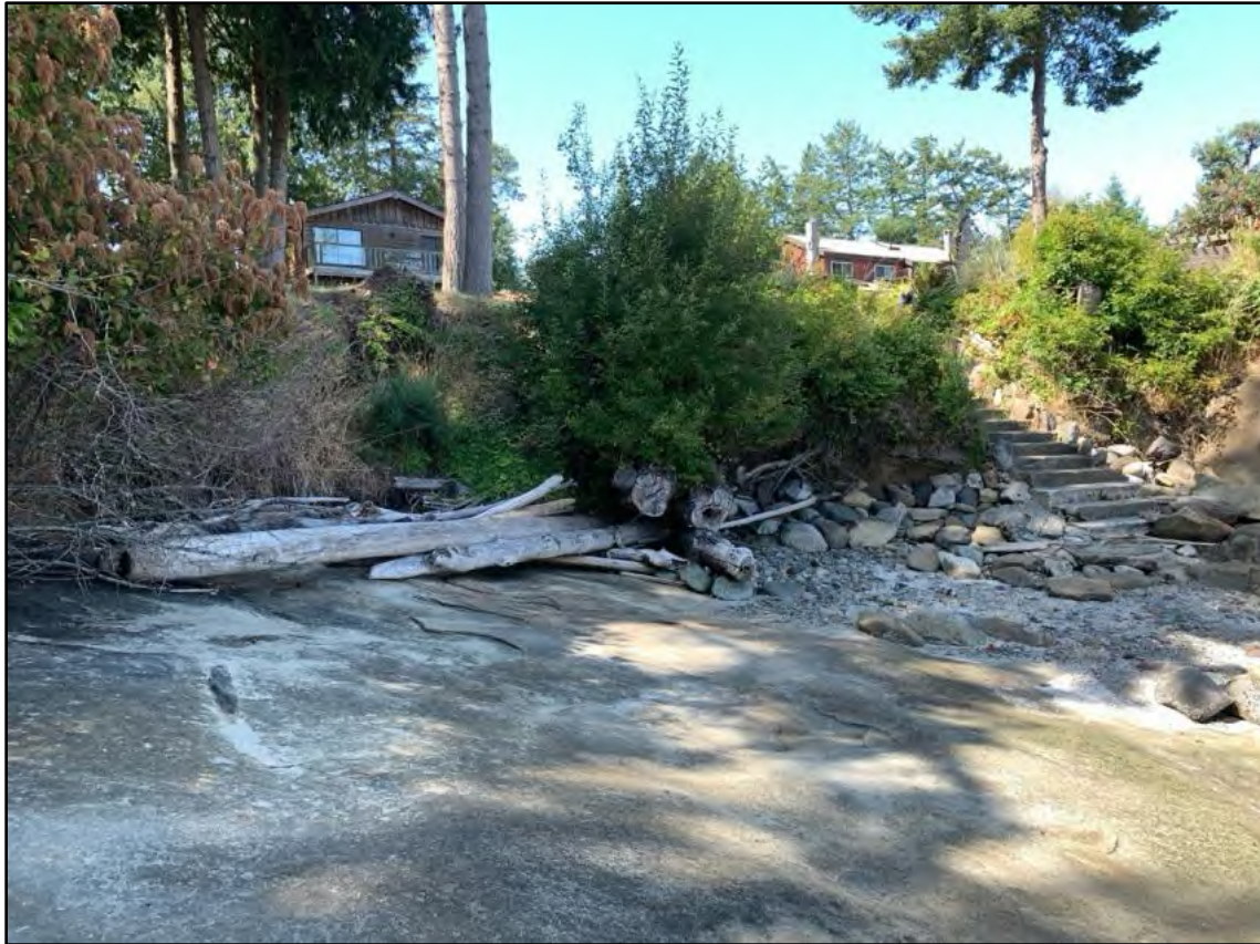
EXISTING STAIRS AND BANK EROSION, LOOKING WEST
