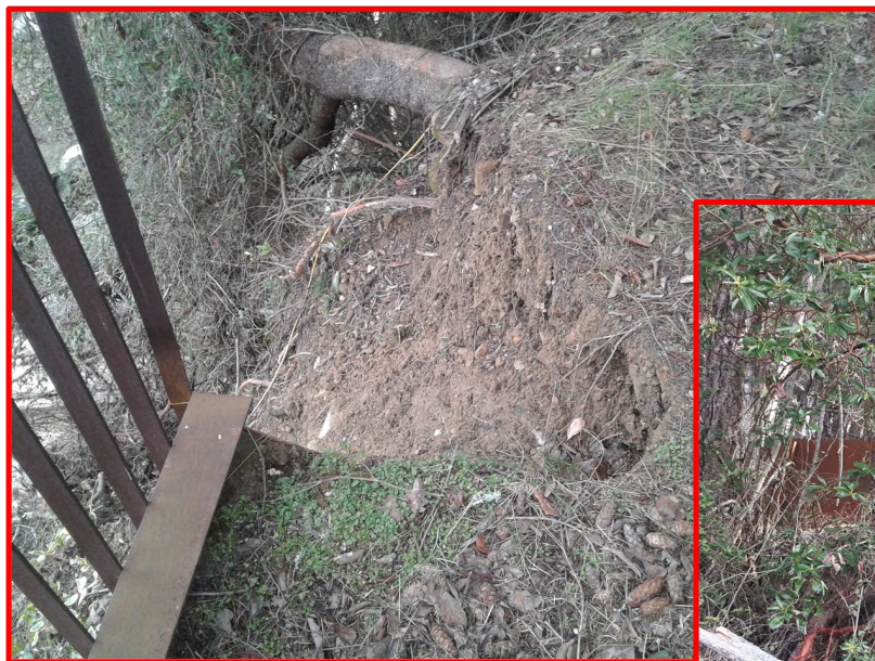
◀ View of eroding section from above
