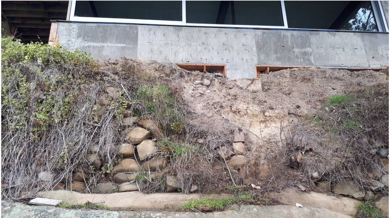
Plate 9. Evidence of erosion along the rock wall near residence at 21455 Porlier Pass Rd., Galiano Island, BC.
