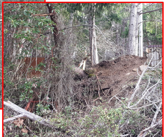
View of eroding section from below ▶
