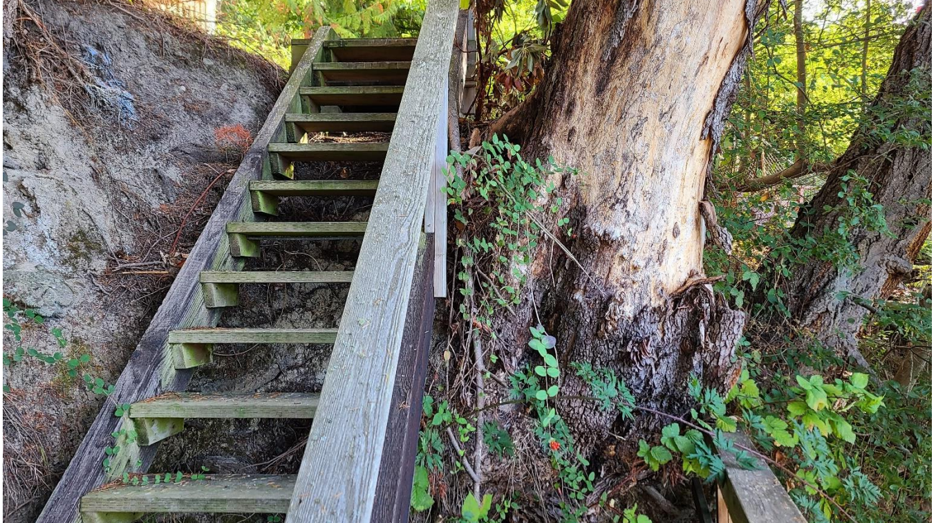
Photo 3: Looking up the beach access stairs from the landing deck. Exposed soil can be seen on the left and the dead arbutus on the right.
