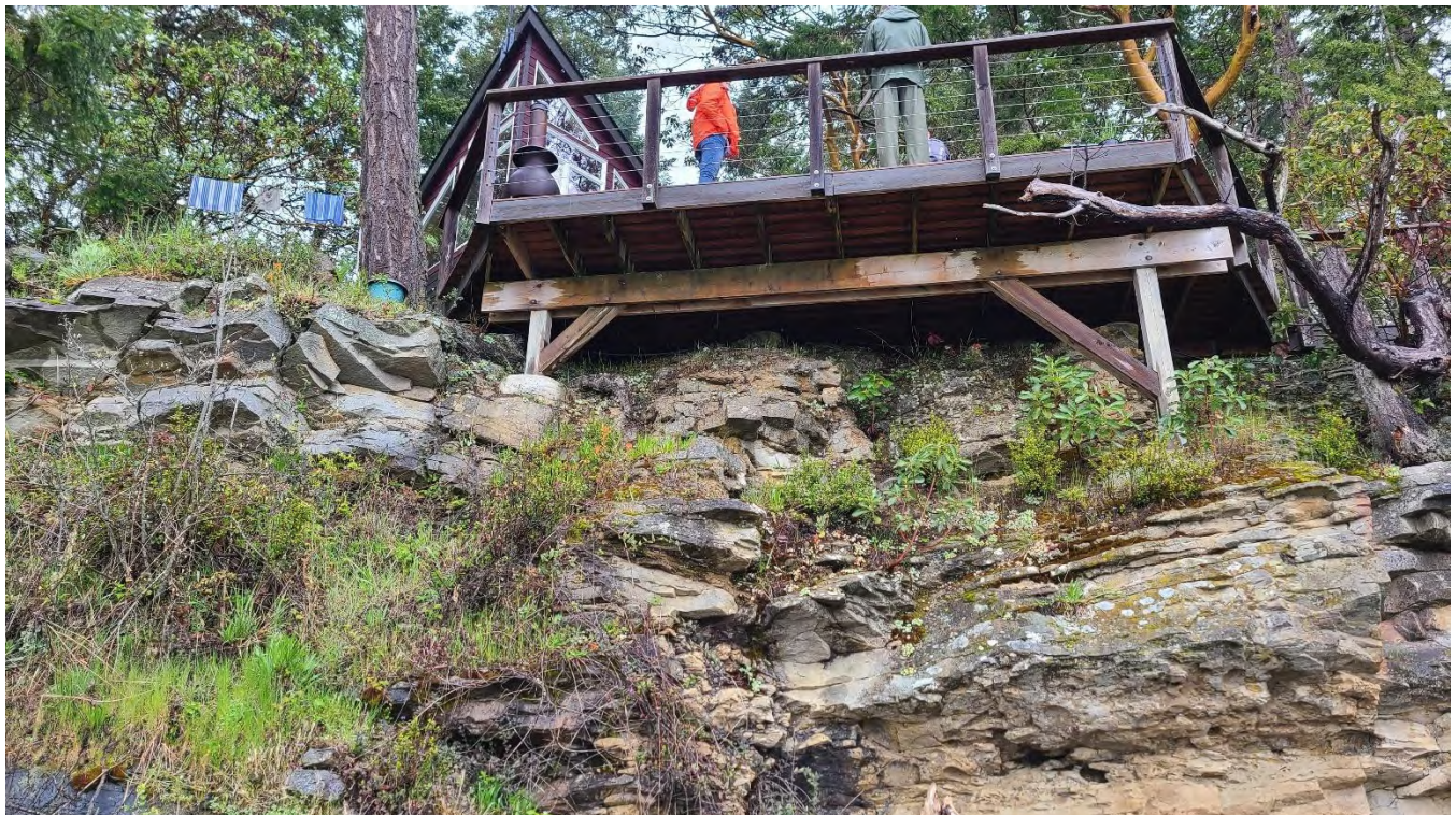
Photo 3: Looking at the cliff and the lower deck from the shore.
