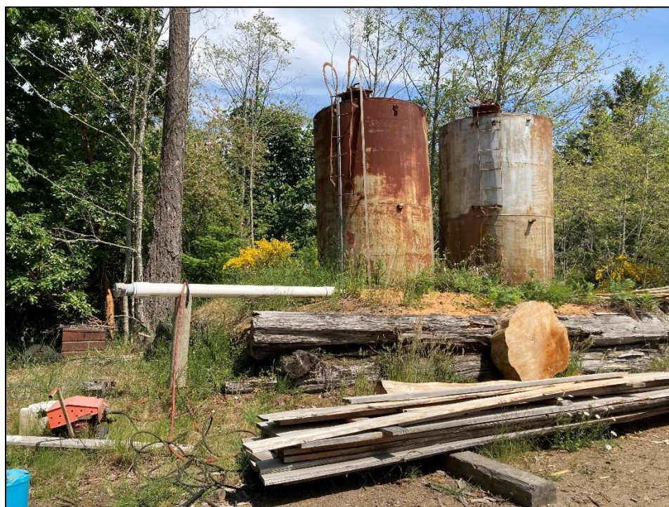
TWO WATER TANKS FOR FIRE EMERGENCIES
