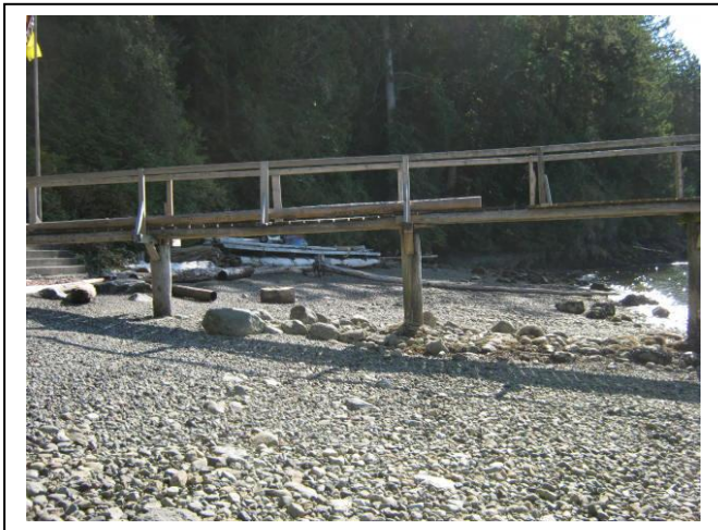
Cobbles at pier footings blocking sediment flow.
