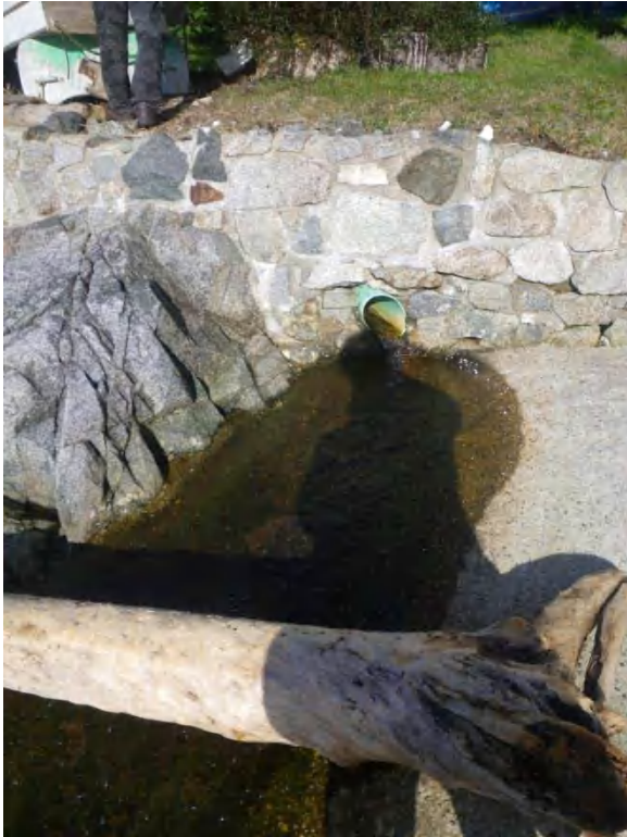
PVC pipe spilling the watershed outlet drainage onto a concrete boat launch located in the intertidal zone.
