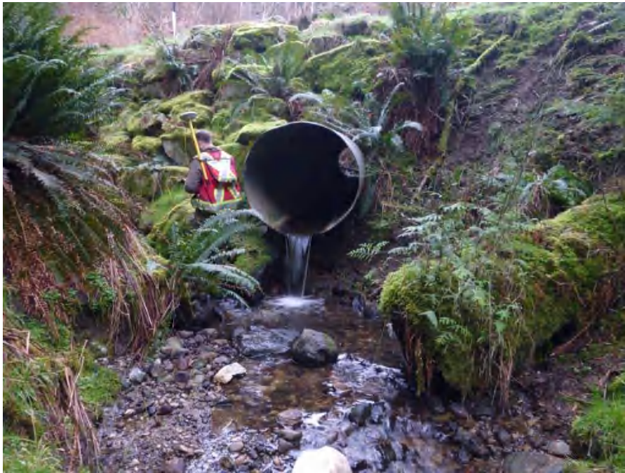
The confluence of tributary 1 with Grennon Creek is represented by a perched culvert which is a barrier to the upstream movement of fish.
