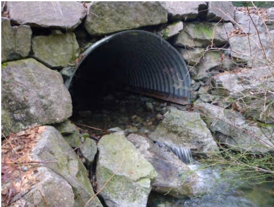
Embedded culvert allows for unimpeded fish passage at the first gravel road crossing.
