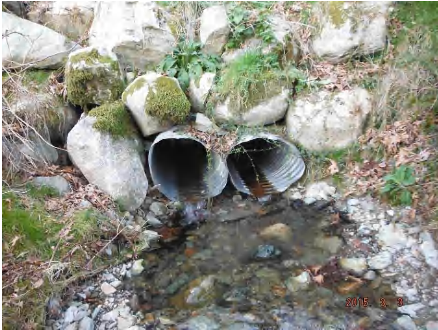
A representative photo of the culverts that have been installed under the road within the residential area. It is unlikely that the culverts represent a barrier to the upstream movement of fish during periods of high discharge.
