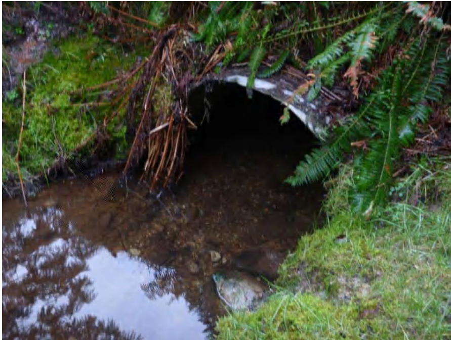
Embedded culvert at the second West Bay Road crossing on Grennon Creek allows for unimpeded fish passage.
