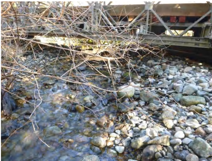
Aggradation of sediment where Whispering Creek flows underneath Mountain Road.
