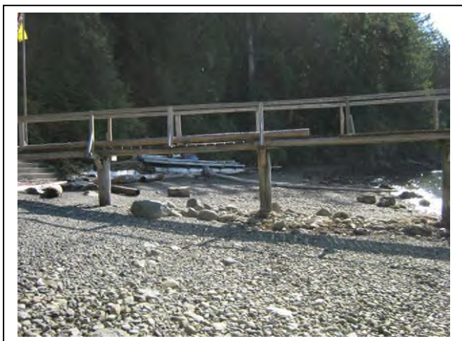
Cobbles at pier footings blocking sediment flow.
