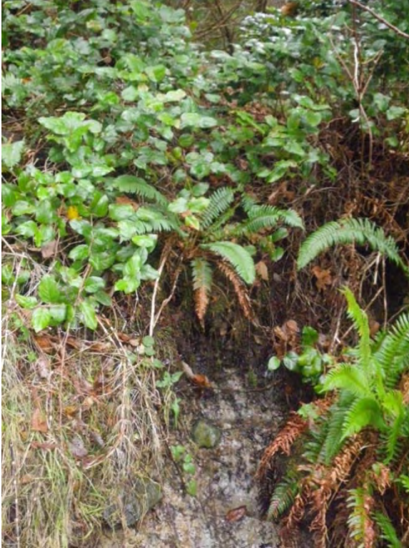
Seepage of water through a steep bank where the outlet drainage meets the intertidal zone.
