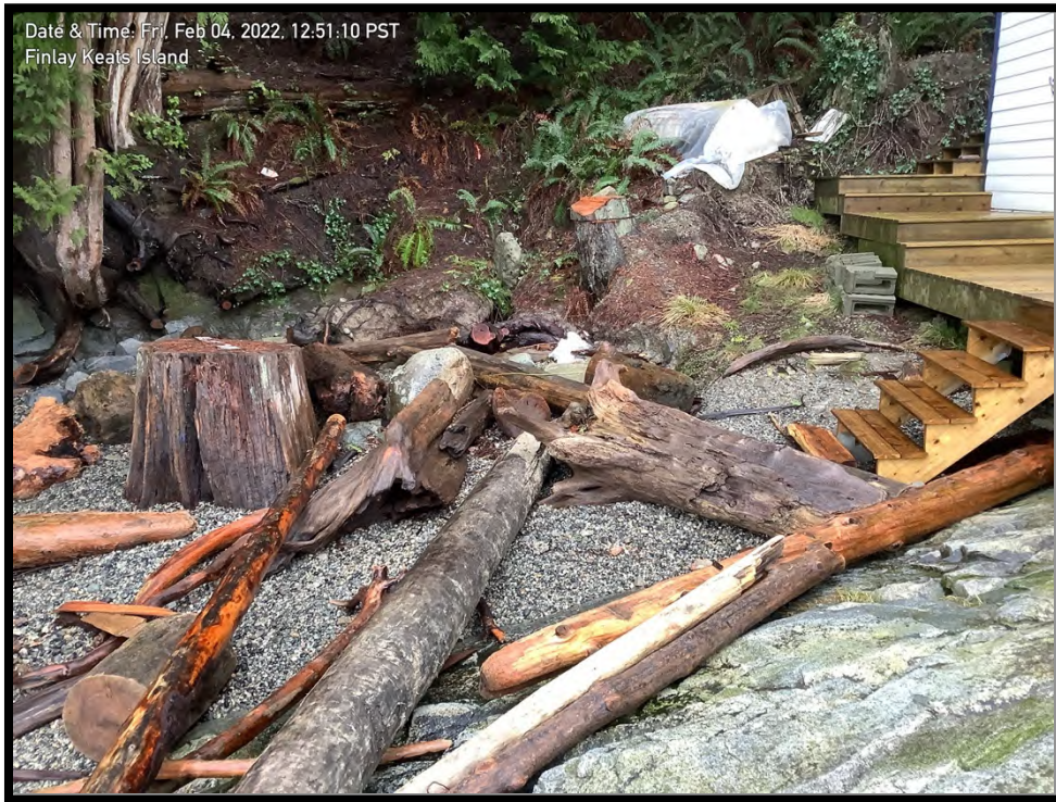
Photo 3: The shoreline fronting the Finlay property at lower tide. The small pocket beach and bedrock sill fronting the home accumulated large wood debris. These materials, during high tide events, with appropriate winds and seas, is battering the home that has no shoreline protection.
