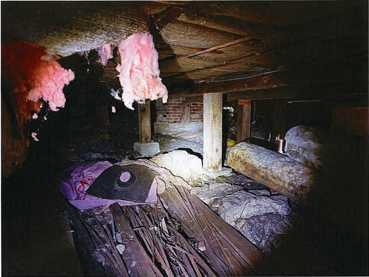
Figure 4: Bedrock outcrops in existing beach house crawl space, existing footings.
