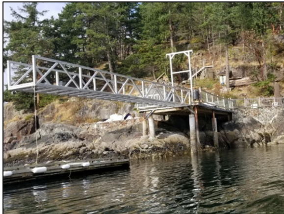
Photo 4. Site 3 float and gangway.
