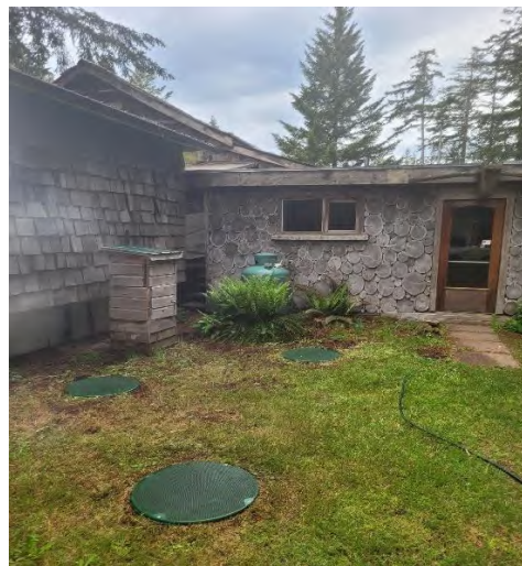
Tank site – control panel in wooden "kiosk" rear left
