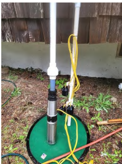
Discharge pump and float switches
