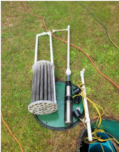
Recirculation pump vault Equipment
