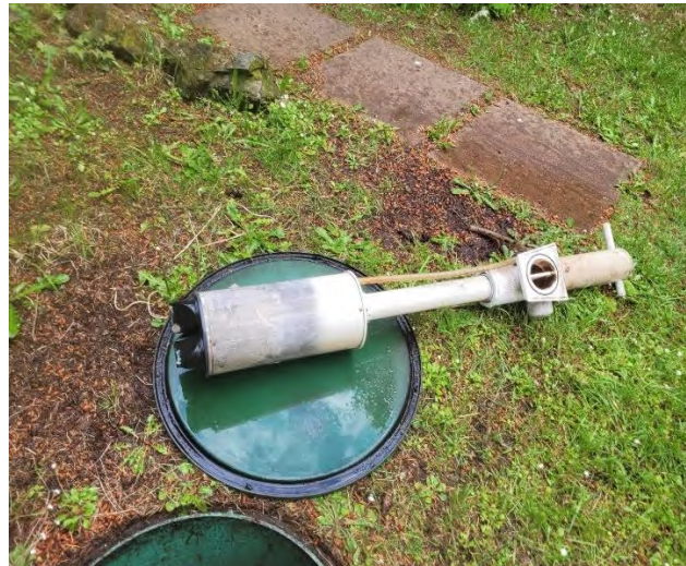
Recirculating ball valve – splits treated effluent flow to discharge basin
