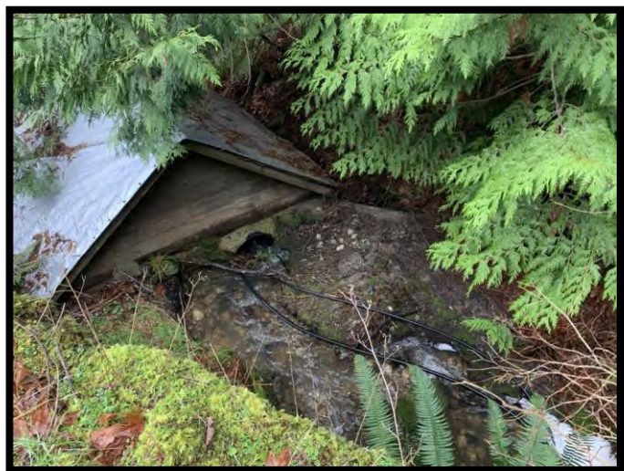
Photo 4. Shed and piping used to divert water to the house, formerly for drinking and then for irrigation.
