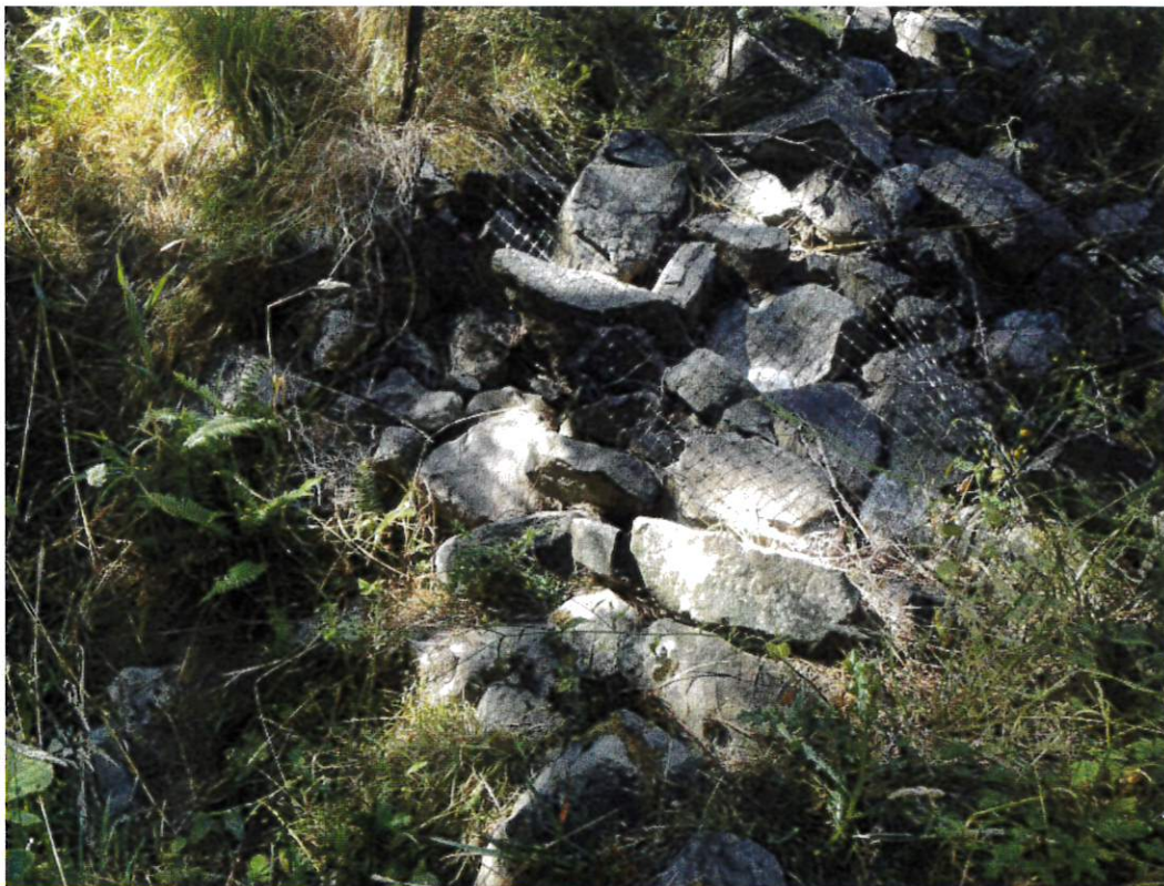
Photo 2. Outlet from the perimeter drains, approximately 5 metres south of the creek channel. Any flows are dissipated by the riprap and flow through a vegetated strip before reaching the creek.
