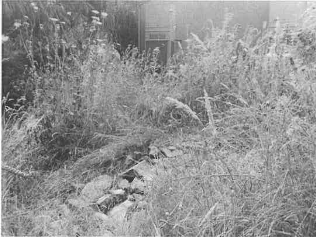
Photo 6. Outlet from the perimeter drains, approximately 5 metres south of the creek channel. Any flows are dissipated by the riprap and flow through a vegetated strip before reaching the creek.
