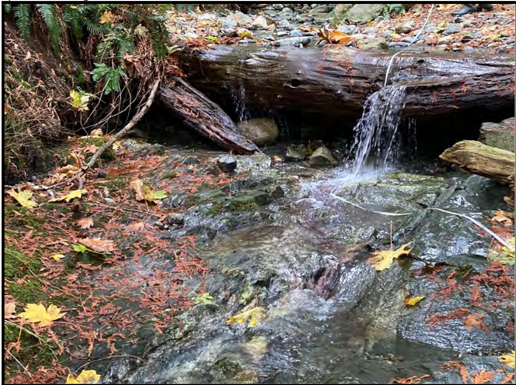
Photograph 6. Upstream view of existing log retaining wall to support existing skid road crossing of Kill Creek.
