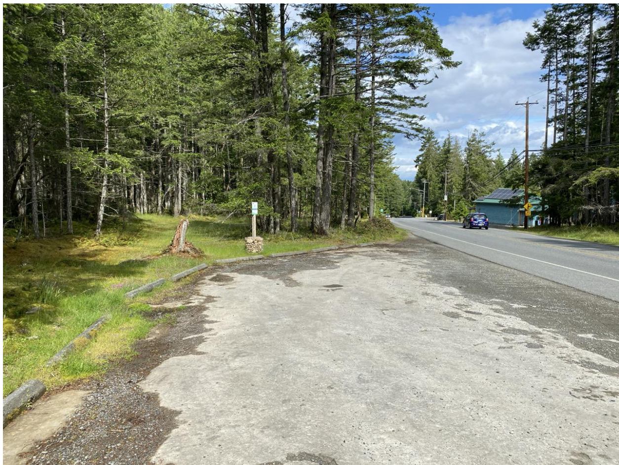
Figure 1. Encroachment damage at McRae NAPTEP Covenant, and the curbs recently installed to deter it. The sign on the rock cairn in the background indicates the approximate property boundary, to which the curbs should be moved in line.
