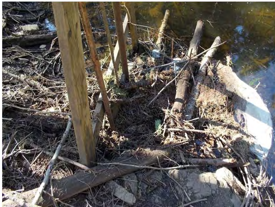
Figure 13. The manmade dam on Trematon Creek. Water flows through a pipe, not visible through the debris. This is a barrier to upstream fish migration.
