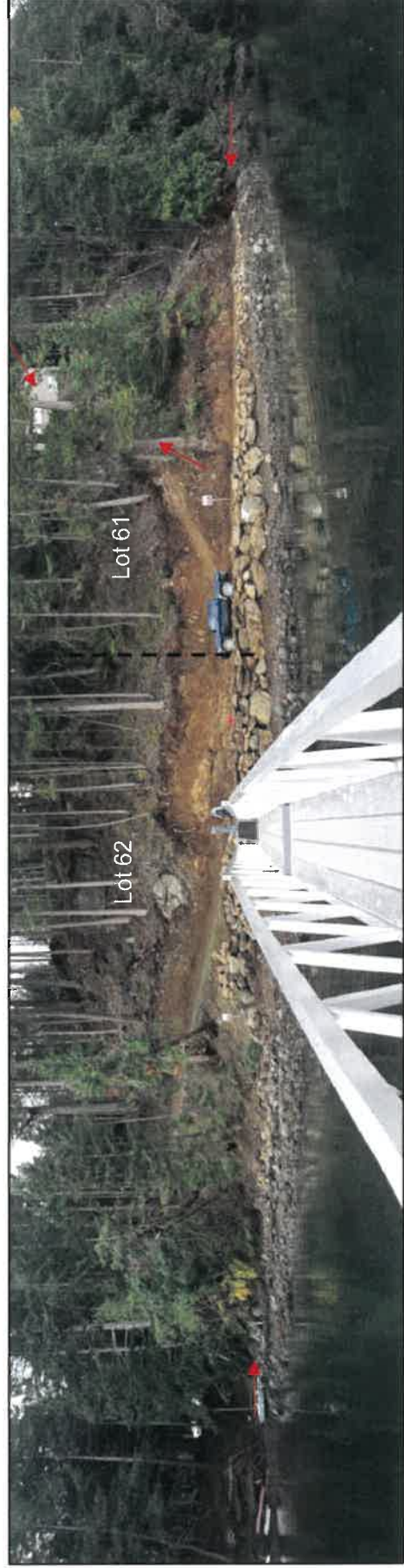
Photo 2. Showing the shoreline taken October 22, 2020 at 9:00am at a 3.6m tide post construction. The rock retaining wall was recently pulled back approximately 2.5m at the toe as it was determined to have encroached past the original Present Natural Boundary of the shoreline. Approximate property line between the two affected parcels is indicated by the black dashed line.
