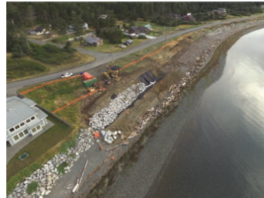
Pictures 3 and 4 depict Low Bank Beaches in Comox, B.C. Rocks and logs are used as a natural approach to slow tidal flows and to prevent erosion.
