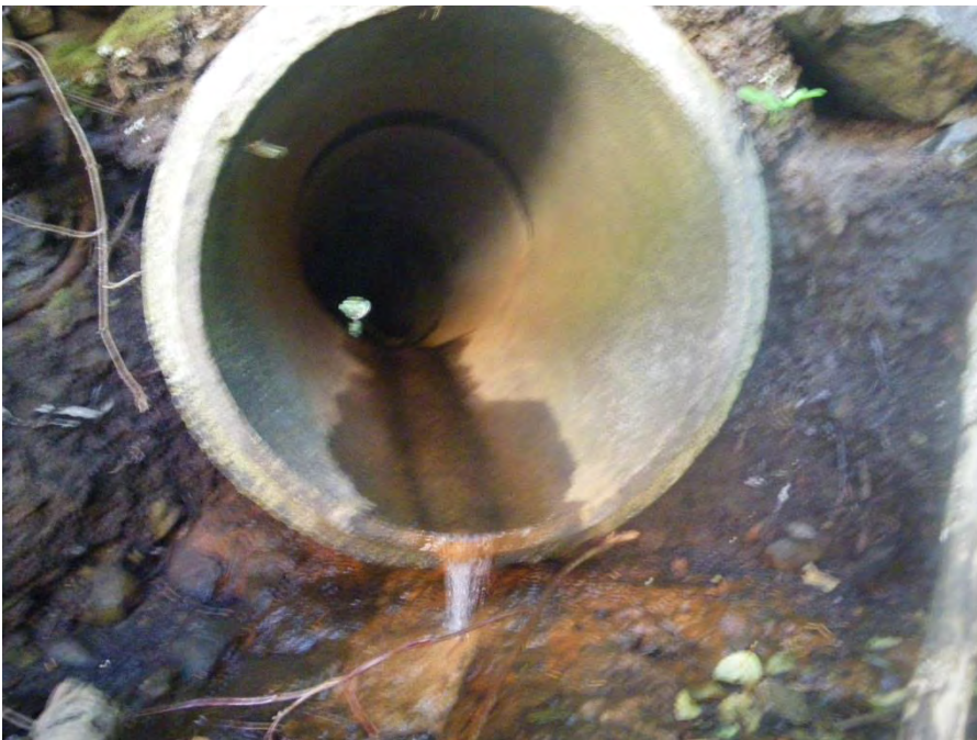
Photo 13. The cement culvert at the outlet of Hadley Creek, near tidewater. It should be noted that this culvert currently represents a barrier (albeit not permanent) to upstream migration by anadromous salmonids.
