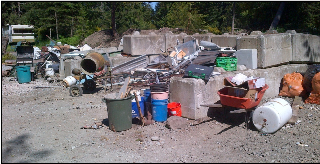
Figure 7: Waste collection bins
