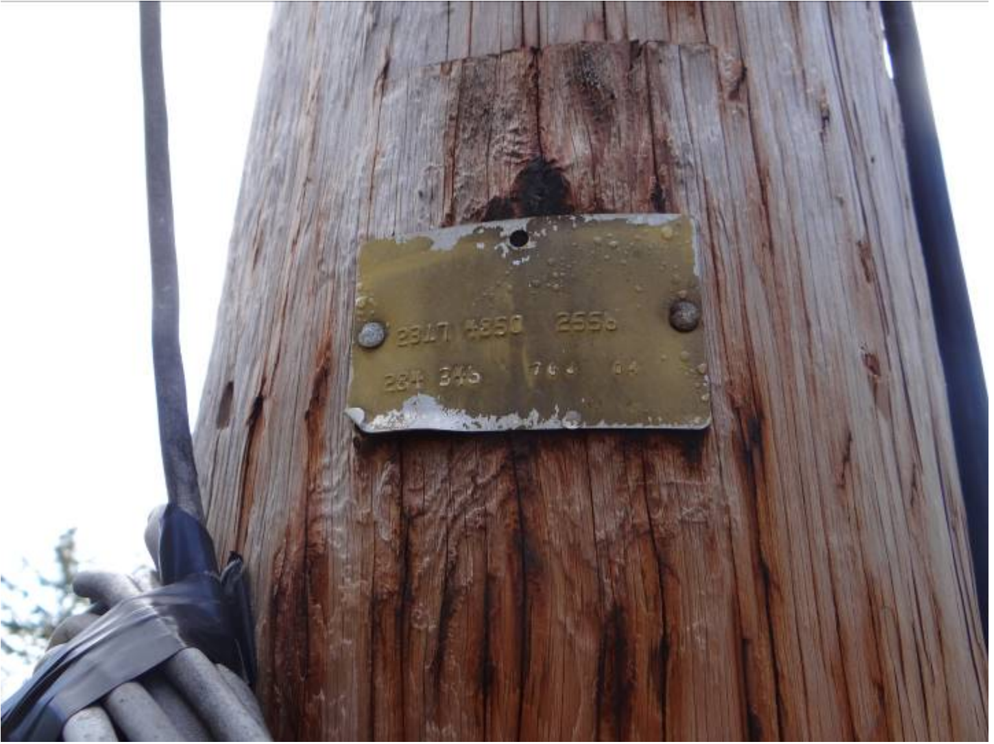
Hydro Service Pole Tag – East of proposed compound
