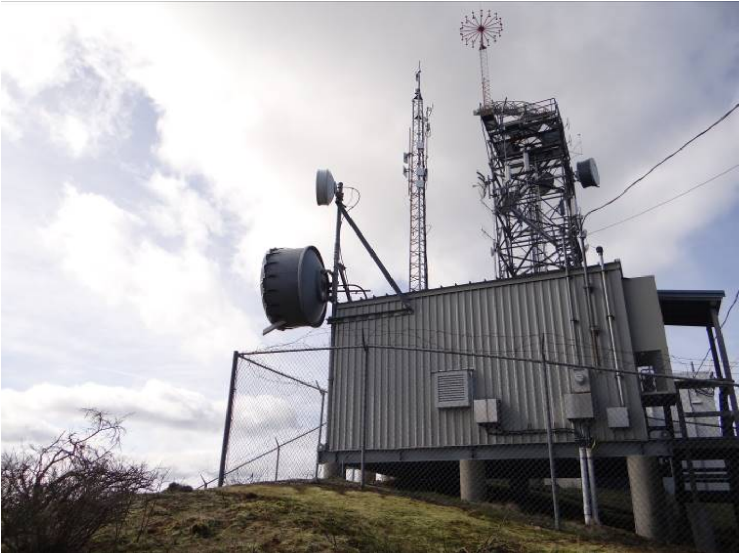
14. Guy Wire Easement Obstructions – Looking North
