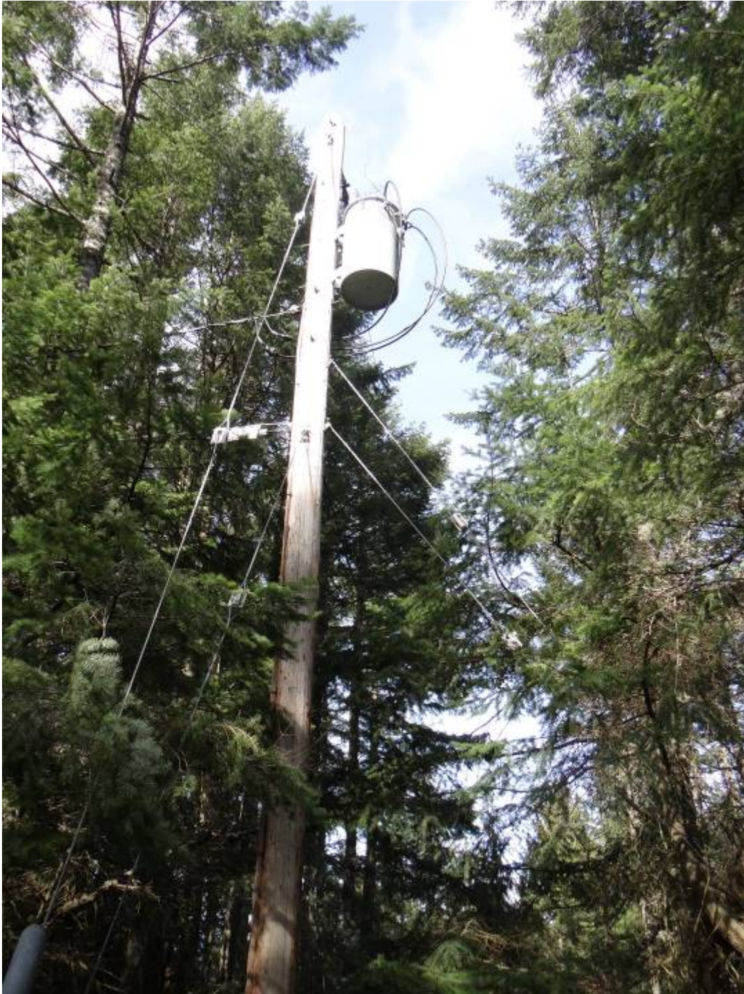
11. Hydro Distribution Pole with 75 KVA Transformer – South of proposed compound
