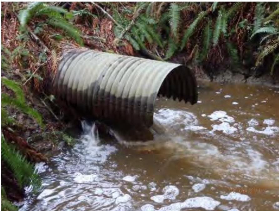
Partially collapsed culvert carrying Horton Creek underneath Horton Bay Road. This culvert will be submerged during high tides.
