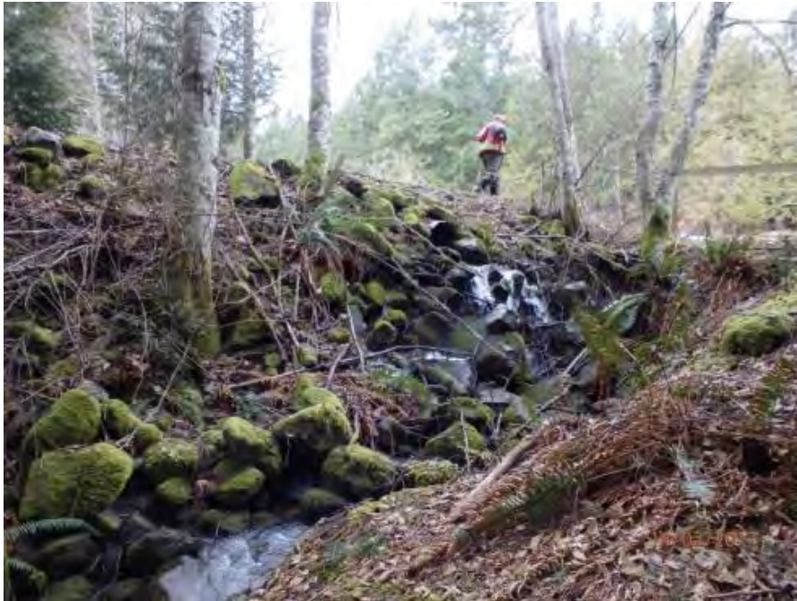
Dam and culvert outlet representing a barrier to upstream fish movement located mid-way through Reach 5 (622 Gallagher Bay Road). This feature is located well above the pond outlet barrier located in Reach 3 and also the perched culvert barrier located at Simpson Road.
