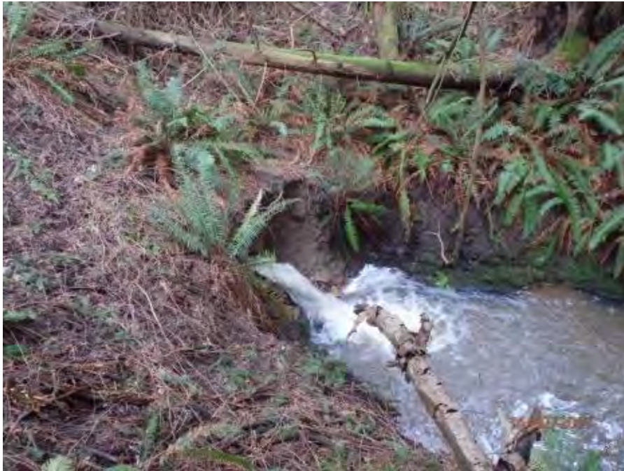
Outflow of perched culvert carrying Horton Creek underneath Simpson Road. This feature represents a barrier to the upstream movement of fish, but is located well above the pond outlet barrier located in Reach 3.
