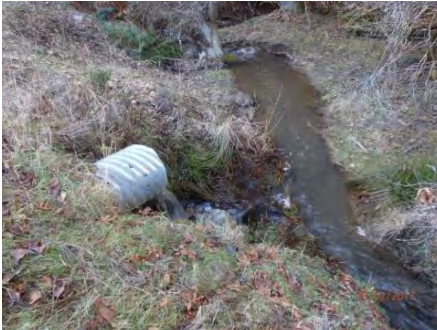
Perched culvert and inflow of ditch flowing along the south side of Merryman Road into Deacon Creek.
