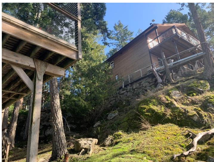
DECK CORNER WITHIN INTERIOR SIDE LOT SETBACK
