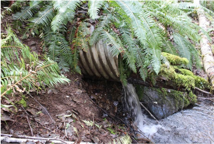
Photo 21. Culvert under trail at Boyle Creek. Culvert is perched and currently blocked with wood.
