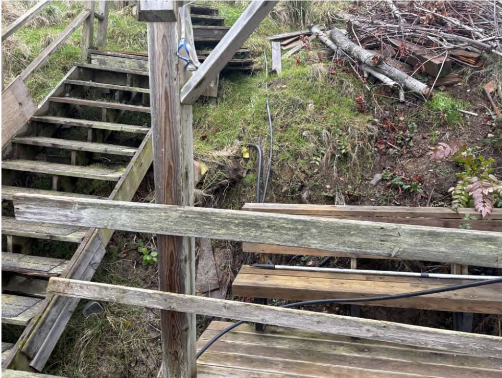
Photograph 5: Soil erosion and landslip visible by the wooden staircase.
