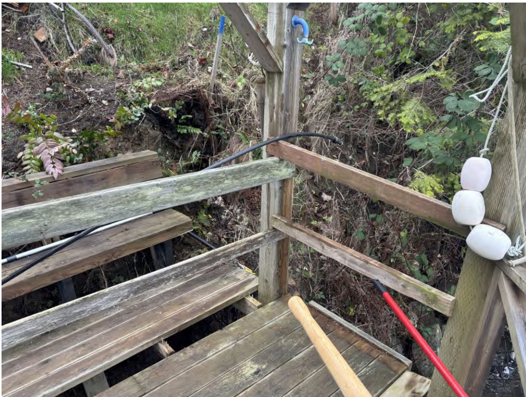
Photograph 6: Soil erosion and landslip visible by the wooden staircase.
