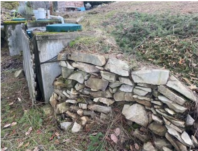
Photo 3. Septic Tanks to be replaced
