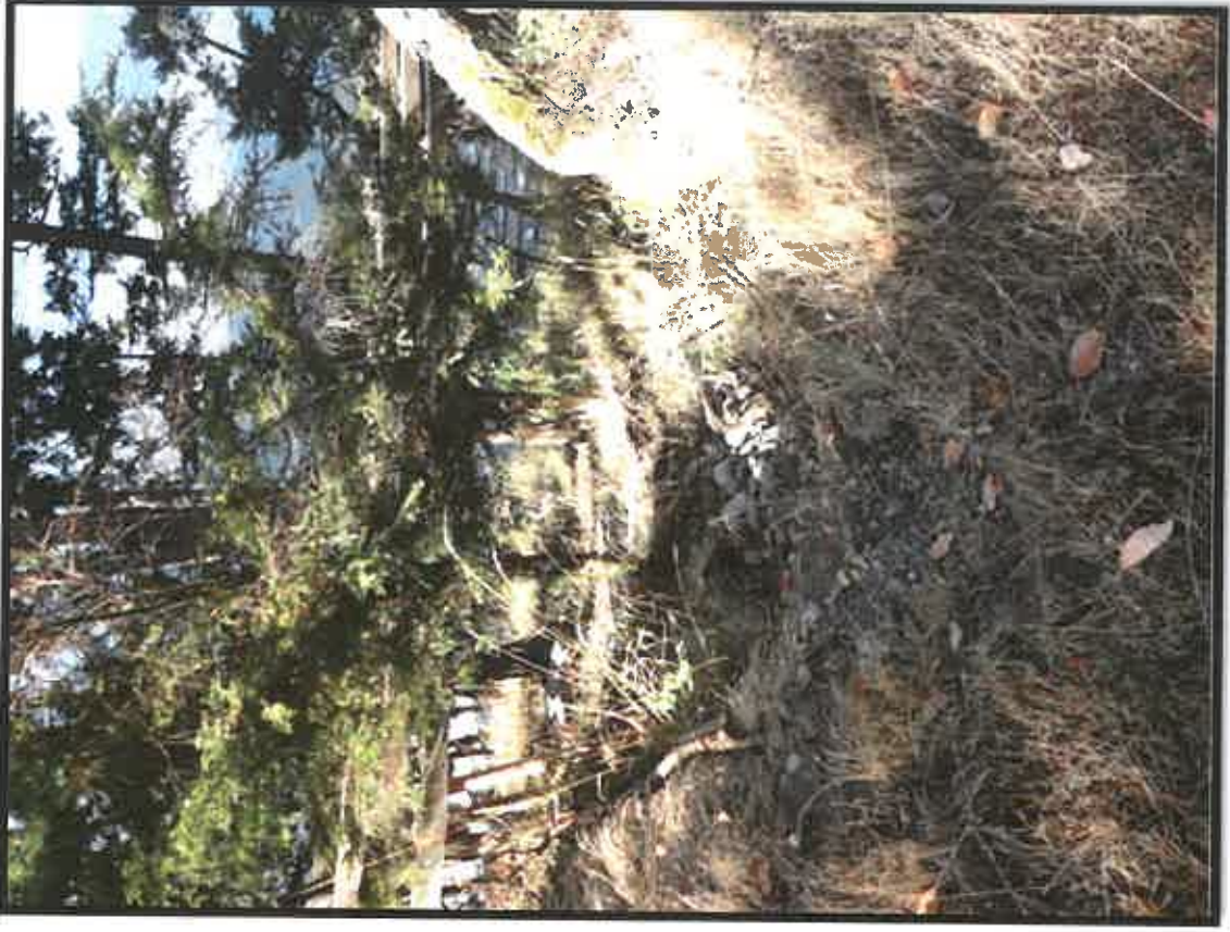
Plate 10: Slope failure originating at top of slope
