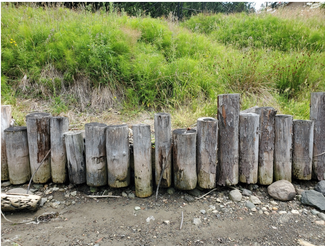
Photo 6. Towards the north end of the site, example of the failing log shoreline stabilization structure and eroding slope behind. Note that the log ends are not embedded into the shoreline substrate.
