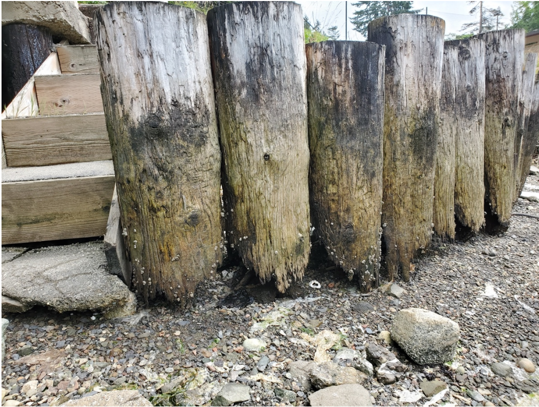
Photo 9. North end of the site adjacent to the dock, example of the failing log shoreline stabilization structure and eroding slope behind. Existing stairs to the shoreline.
