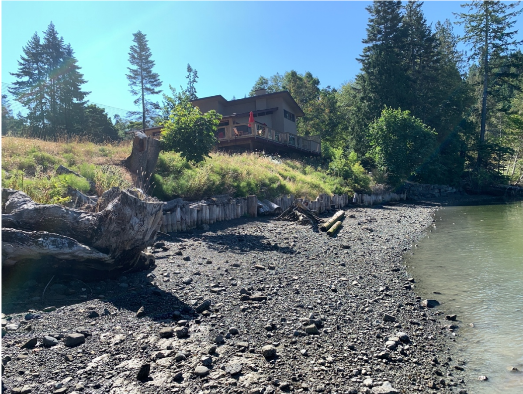
Photo 1. Looking south along the shoreline at failing log shoreline stabilization structure and eroding slope behind.
