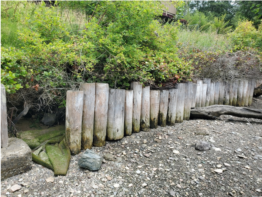
Photo 7. Towards the southern end of the site, near the house, remnant native vegetation on the overhanging slope, revealing erosion and old carpeting used in the original structure.
