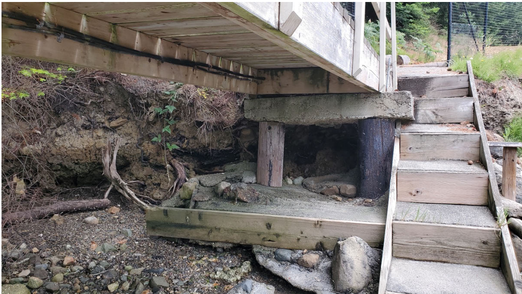
Photo 10. North end of the site at the dock and undercut eroding bank, with existing stairs to the shoreline.
