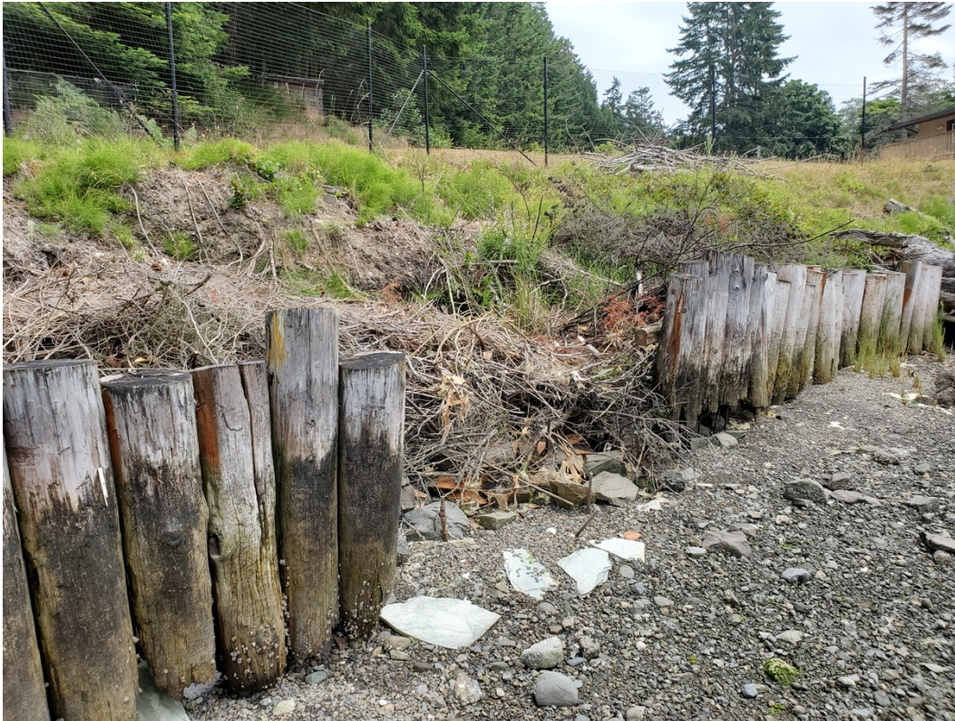
Photo 5. Towards the north end of the site, example of the failing log shoreline stabilization structure and eroding slope behind.
