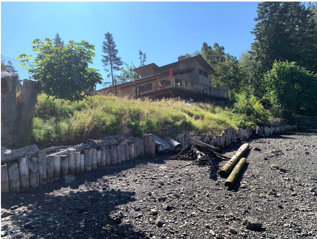
Photo 2. Looking south along the shoreline at failing log shoreline stabilization structure and eroding slope behind.
