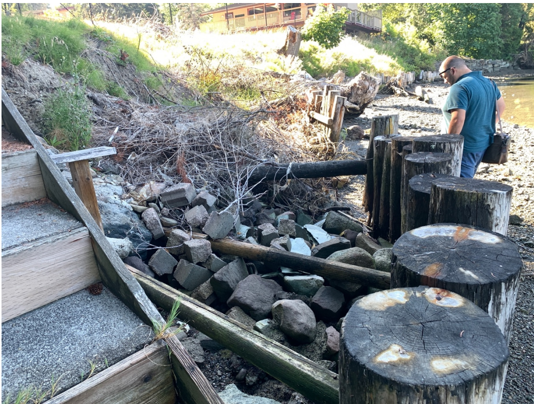
Photo 8. North end of the site adjacent to the dock, example of the failing log shoreline stabilization structure and eroding slope behind, with materials placed over the years to try to stop the erosion. Existing stairs to the shoreline.
