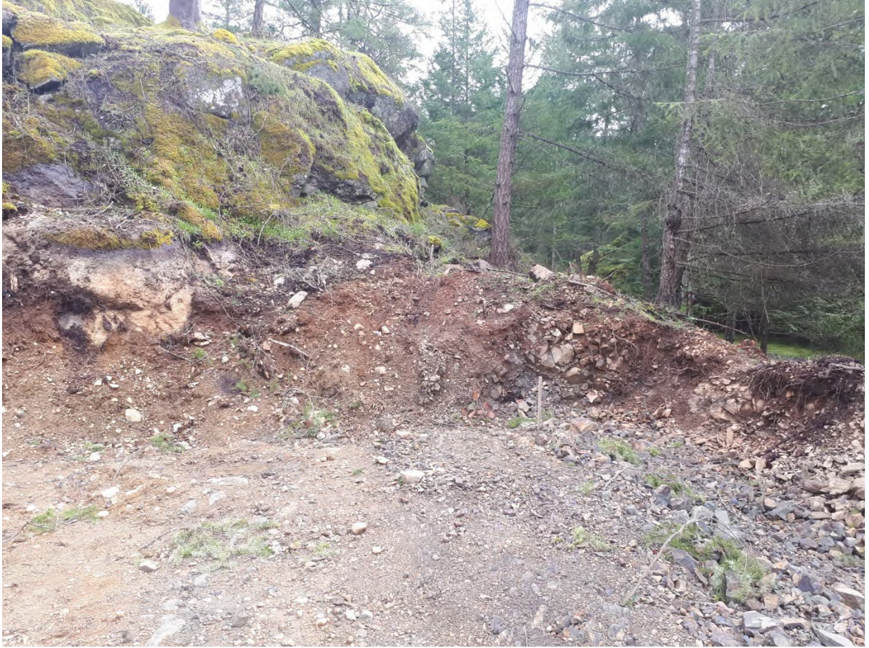
Figure 4. Close up of area needing remediation (slope leveling and replanting).
